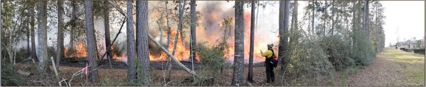
Forest Management in the Wildland/Urban Interface continues to grow. Here a boundary service road was utilized as a fuel break for implementing a prescribed burn in the timber stand; while the mowed grass on the right created a fuel break between the forest and a neighborhood. Photo©Texas Forest Service (TFS).
